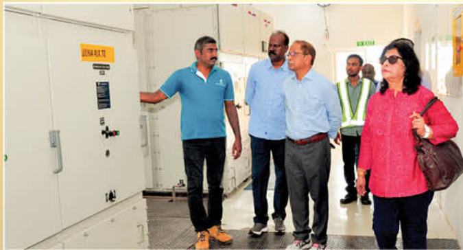
A view during the IEM visit to 50 MW Solar Power Project, Kasaragod
