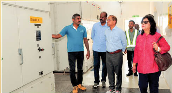
A view during the IEM visit to 50 MW Solar Power Project, Kasaragod
