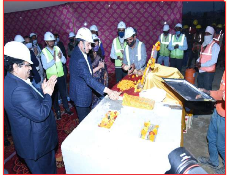
Sh. D. V. Singh, CMD, THDCIL at commencement of Boiler Erection Unit # 1 at Khurja STPP
