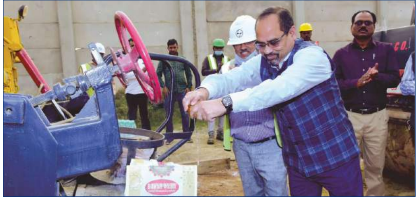
Sh. J. Behera, Director (Finance) inaugurating Pre Assembly of Ceiling Girders of Boiler-1
