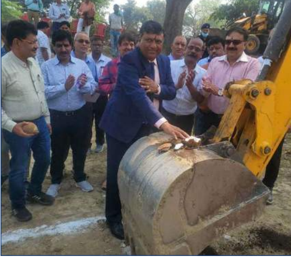
A view of Chairman and Managing Director inaugurating 02 Nos Sedimentation Tanks at Mundakhera, Bulandshahar for KSTPP
