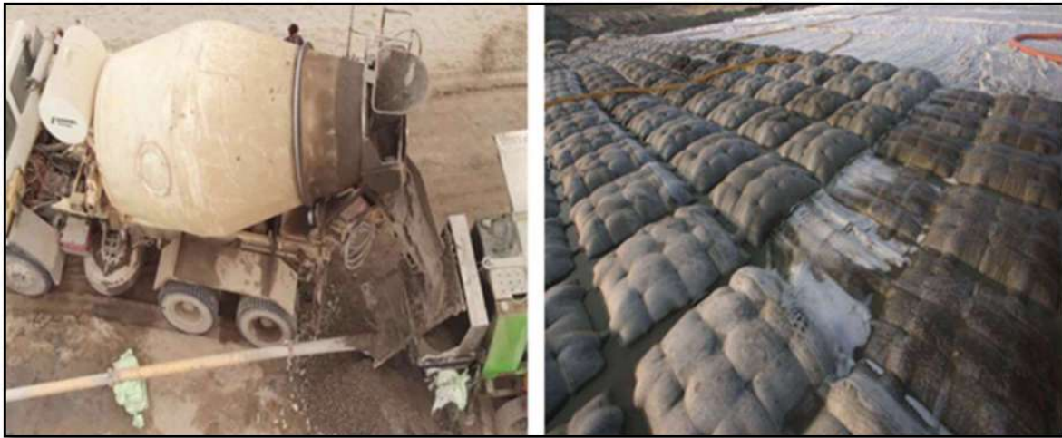
Fig.- (a) Image showing the process of concrete filling (b) Image showing installed Articulating Grouted Concrete Mattress after concrete filling
