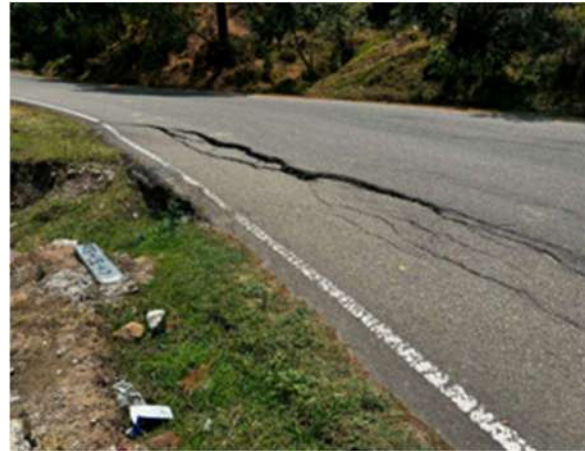
Fig. Prominent Cracks developed on the pavement
