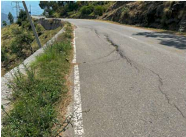
Fig. Initial subsidence observed on the Road
