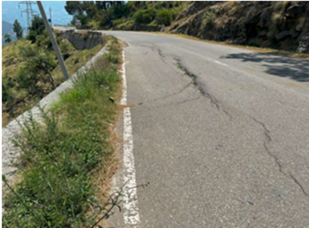
Fig. Initial subsidence observed on the Road
