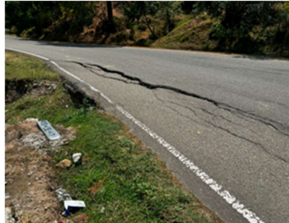
Fig. Prominent Cracks developed on the pavement
