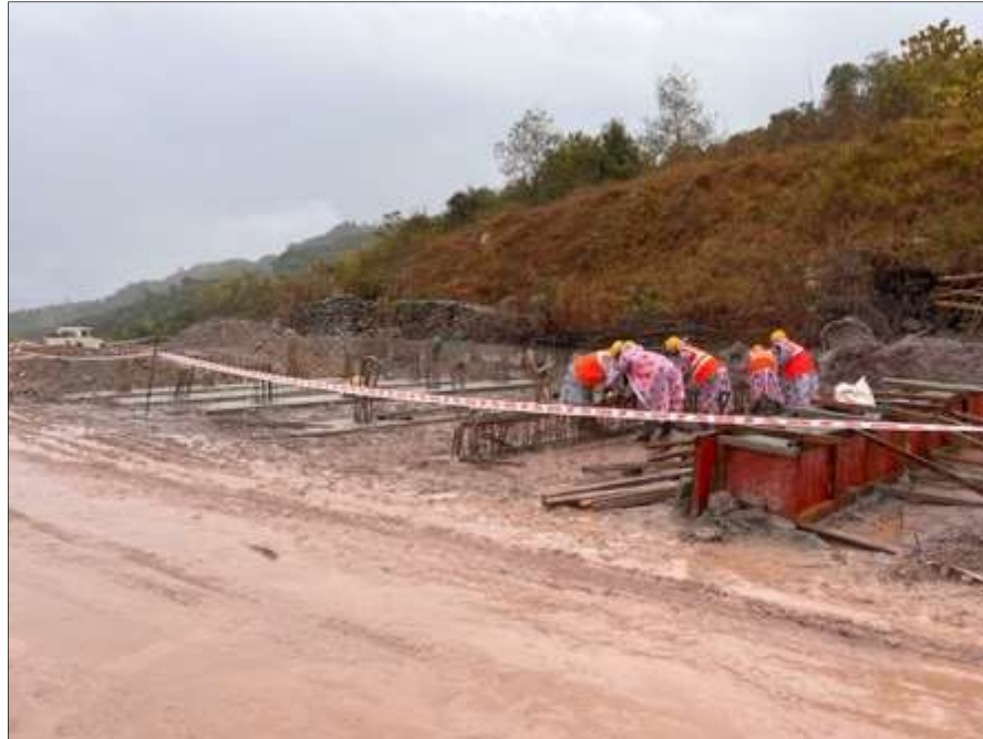
Fig. The proposed arrangement in construction at one of the site in Arunachal Pradesh along NH-513 (Pasighat-Yingkiong)
