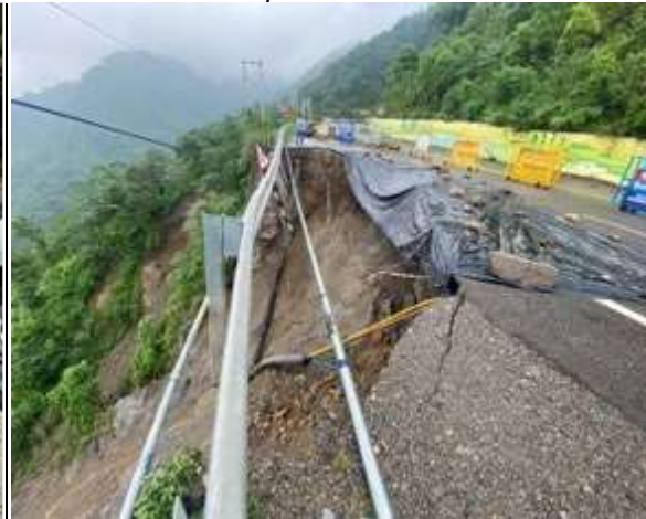
Fig. Loss of valley side portion of the pavement
