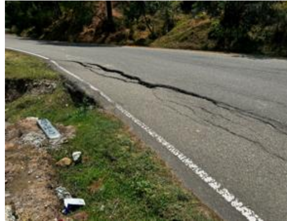
Fig. Prominent Cracks developed on the pavement
