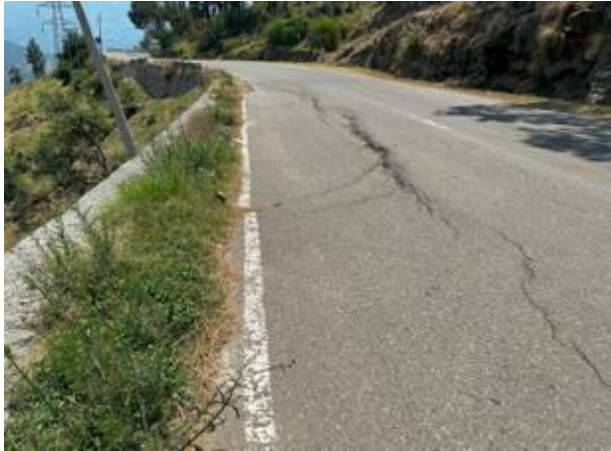
Fig. Initial subsidence observed on the Road
