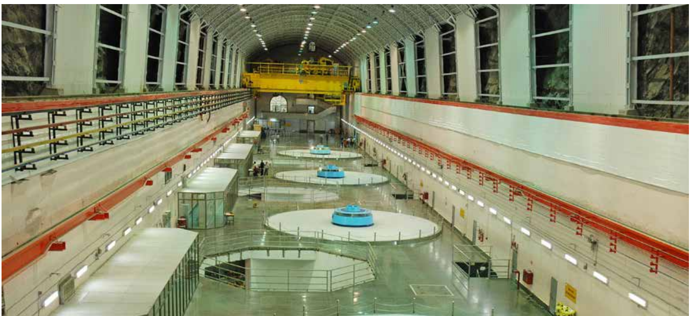
A view of underground Power House of Tehri HPP (1000 MW)
