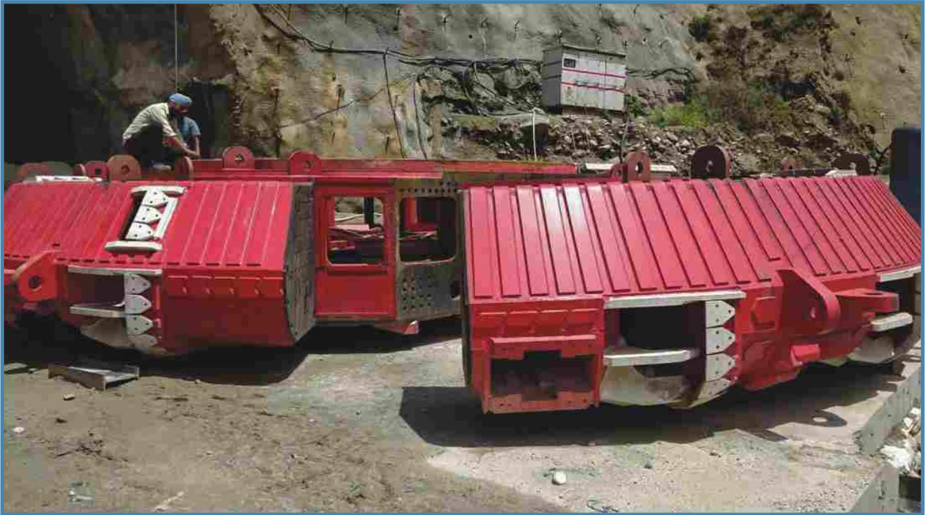
Assembly of Tunnel Boring Machine at Vishnugad Pipalkoti HEP (444 MW) in Progress
