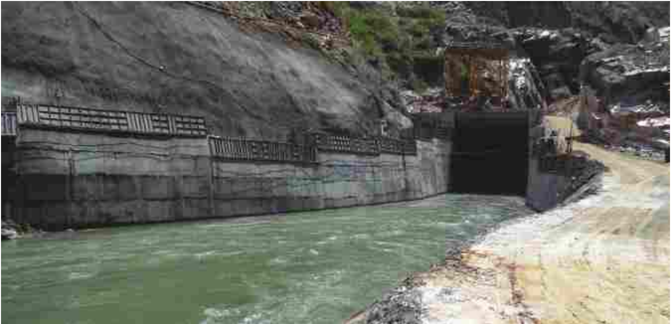
River Alaknanda diverted through Diversion Tunnel on 02.04.2018 at Vishnugad Pipalkoti HEP (444 MW)
