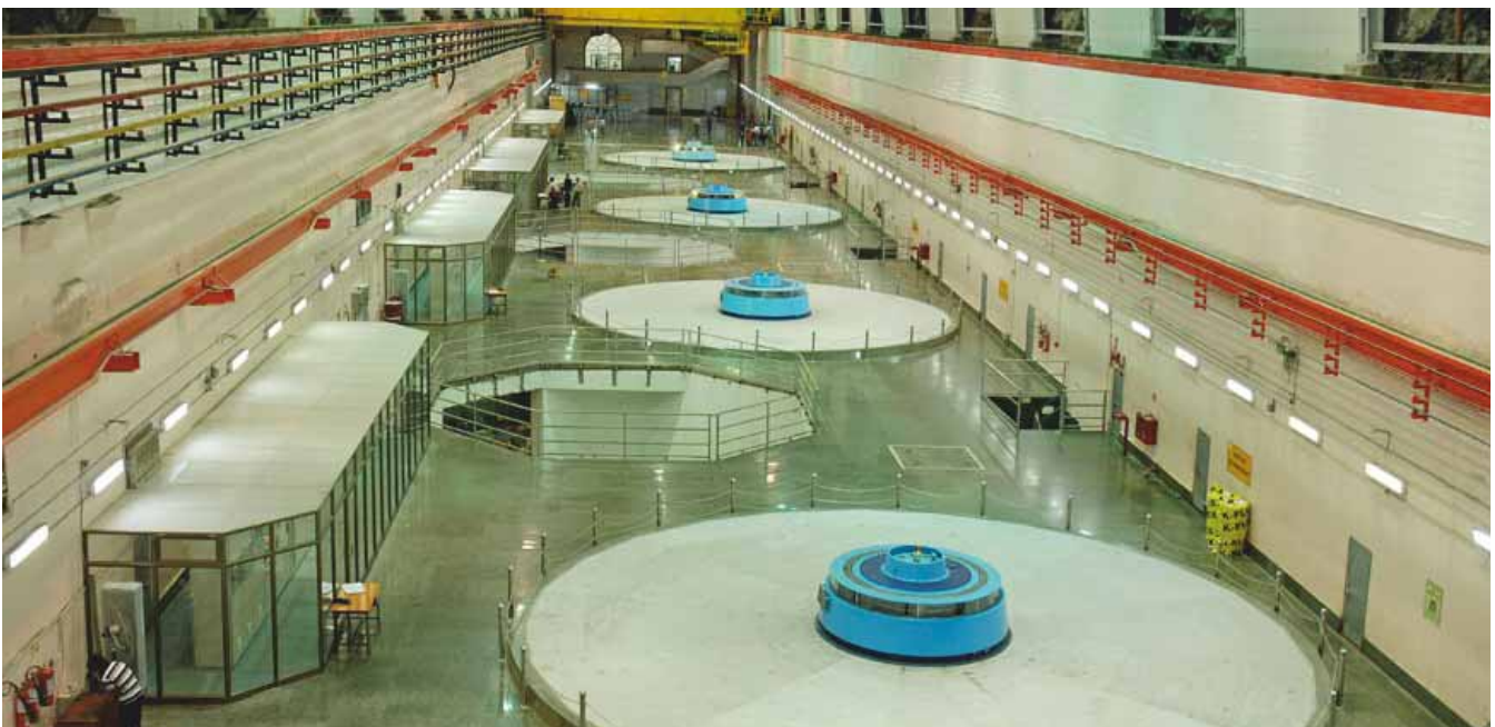
A view of underground Tehri Power House
