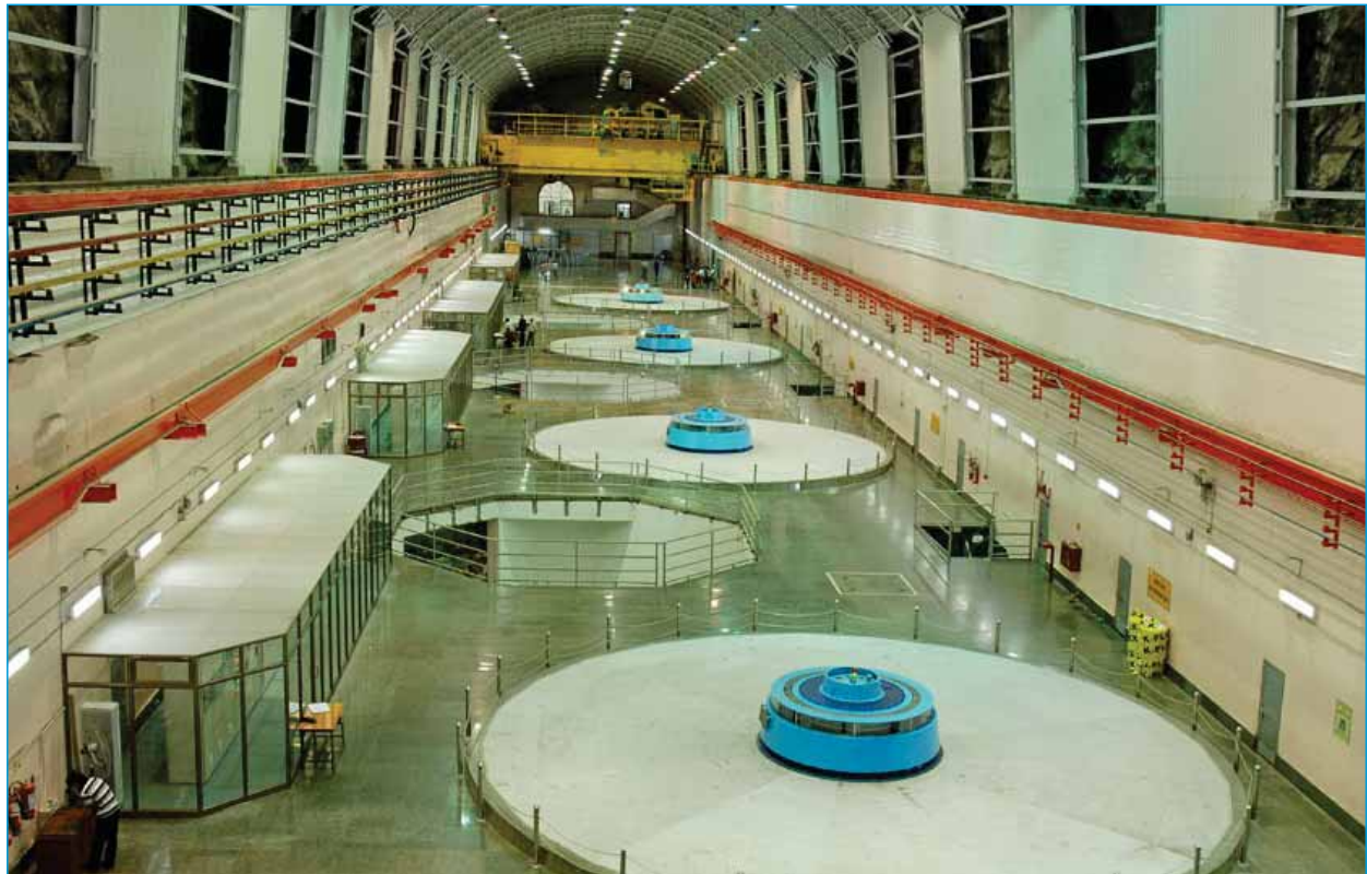
A view of Underground Power House of 1000 MW, Tehri HPP
