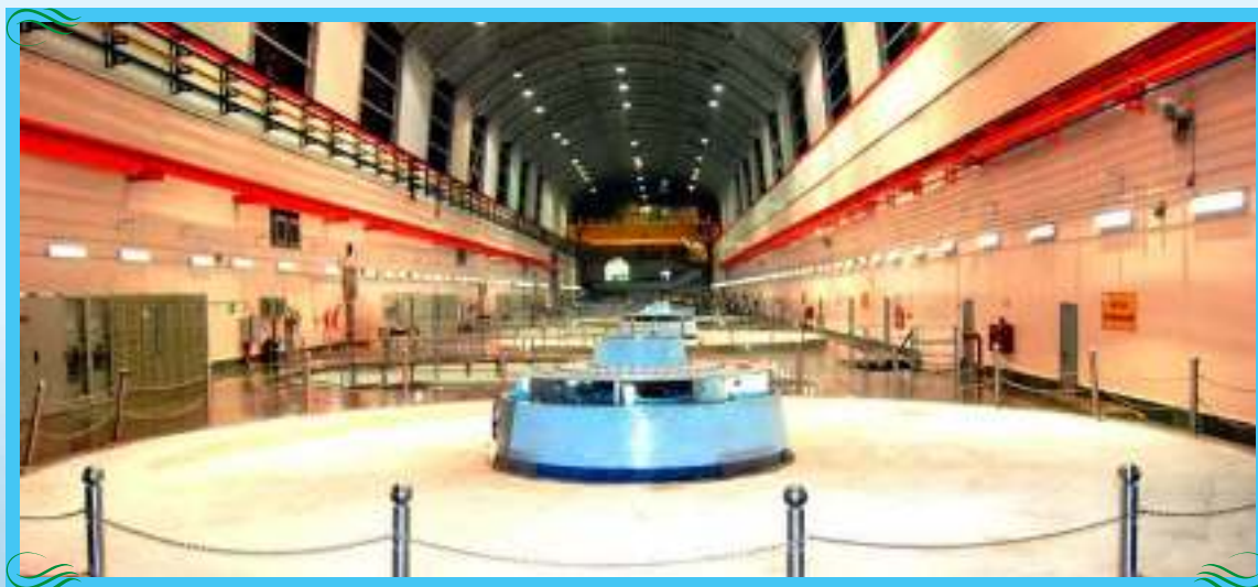
A view of Underground Power House of 1000 MW, Tehri HPP
