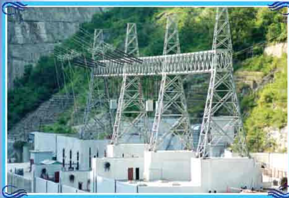
Power Evacuation from Tehri HPP
