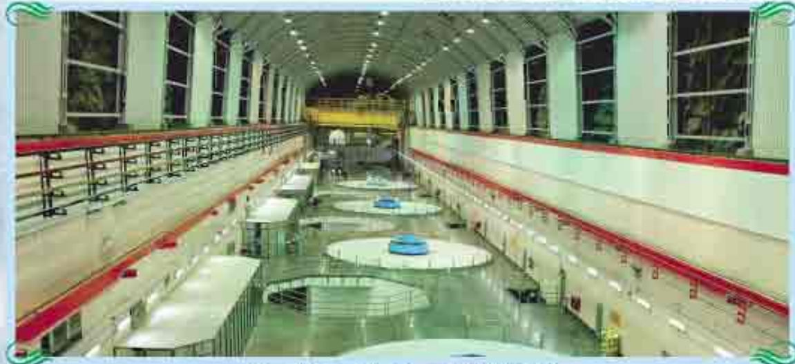
A view of Underground Power House of 1000 MW, Tehri HPP.
