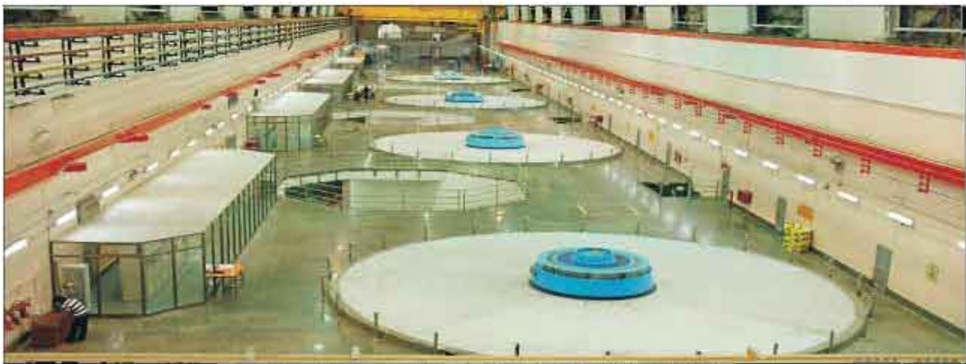
A view of underground Power House of 1000 MW, Tehri HPP
