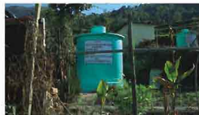
Water Harvesting installed by SEWA THDC at Kathuli village in Tehri an amount of ₹ 1.95 Cr. at New Tehri Town for the benefit of the students of SC/ST communities.
