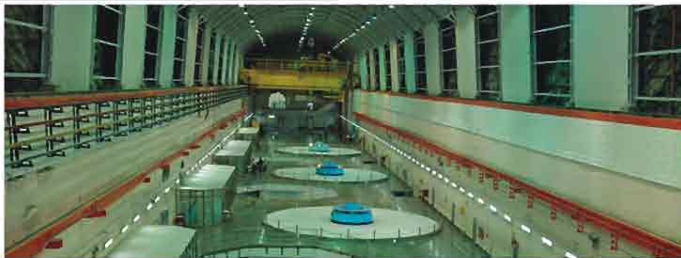
A view of underground Power House of 1000 MW Tehri HEP
