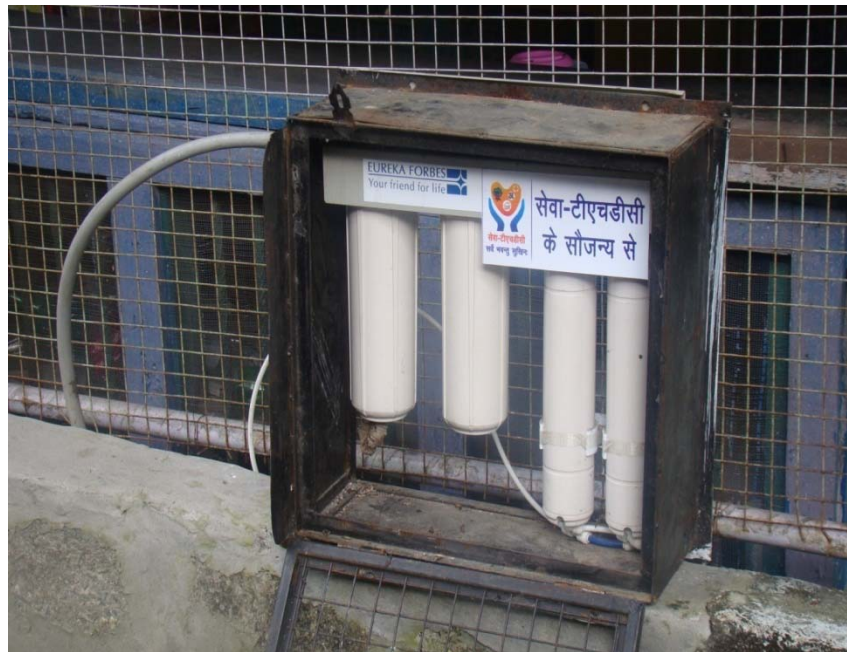
UNIT INSTALLED AT MAIN MARKET PAKHI (GAURAD GANGA) ON NH-58 ADJACENT TO DGBR OFFICE UNDER JOSHIMATH TEHSIL
