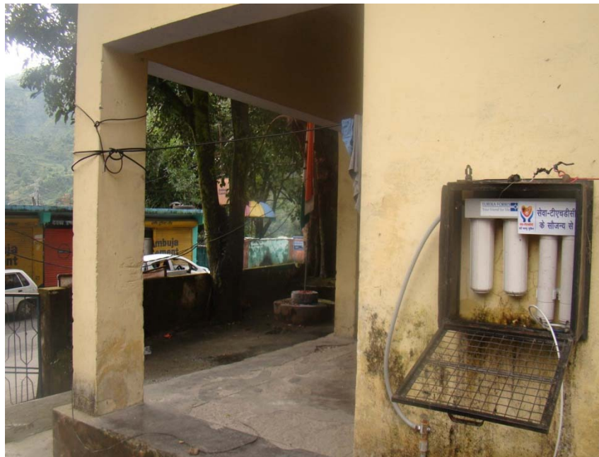
UNIT INSTALLED AT MAIN MARKET NAND PRAYAG ON NH-58 IN PREMISES OF POLICE THANA, NAND PRAYAG UNDER CHAMOLI TEHSIL
