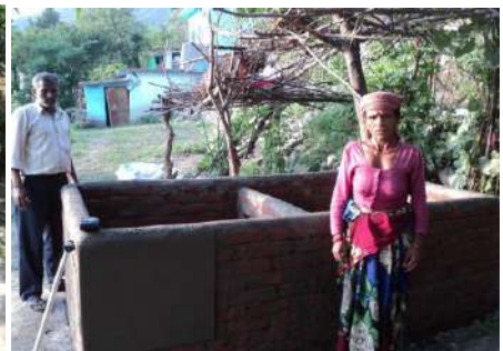
Completed work of Vermin Compost Pit – Beneficiary Smt. Deepa Devi, Village Gandoli – Photo on 23 rd June 2018
