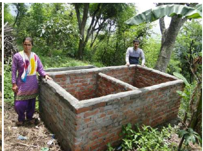
Completed work of Vermin Compost Pit – Beneficiary Smt. Hansa Devi, Village Mundoli (Nelda)– Photo on 25 rd June 2018
