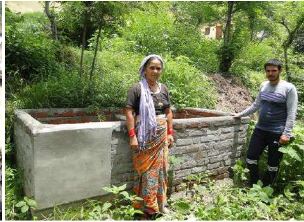
Completed work of Vermin Compost Pit – Beneficiary Smt. Seela Devi, Village Mundoli (Nelda)– Photo on 25 th June 2018
