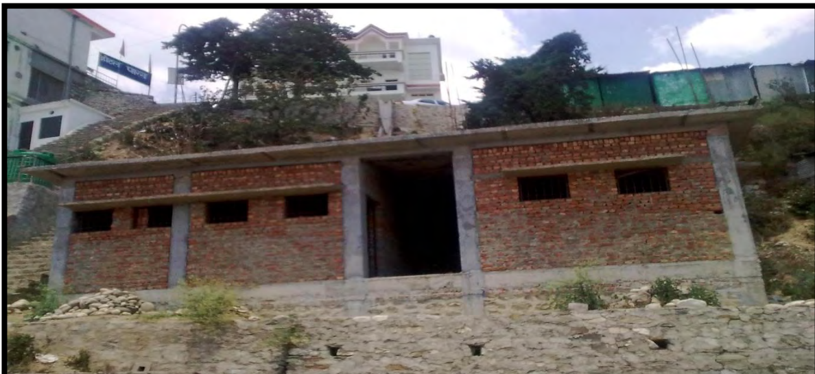
View of under construction of toilet complex at New Tehri Town, Tehri
