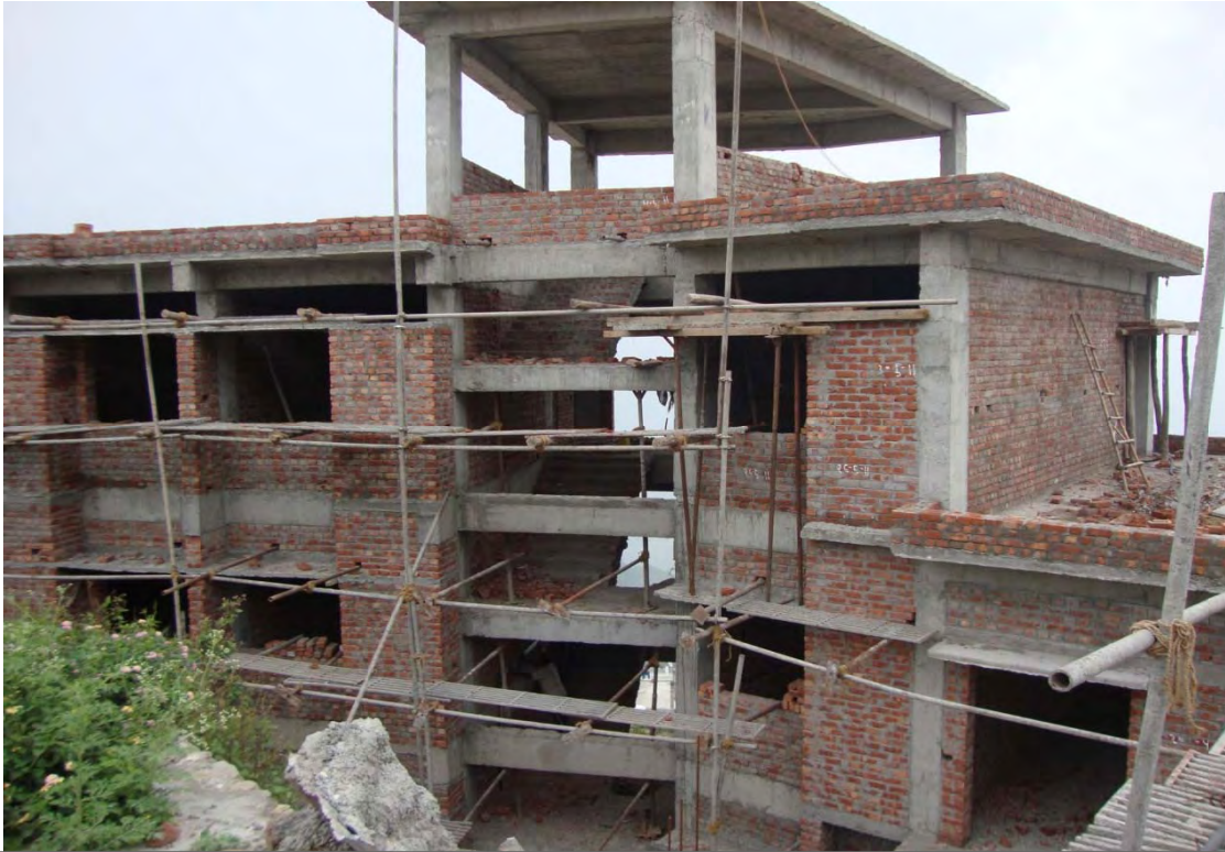
A view of under construction SC/ST Hostel at New Tehri Town (NTT)
