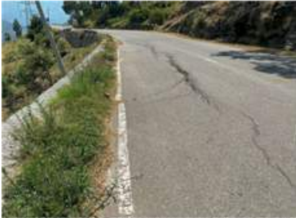
Fig. Initial subsidence observed on the Road
