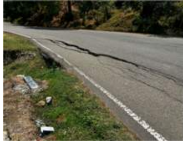
Fig. Prominent Cracks developed on the pavement
