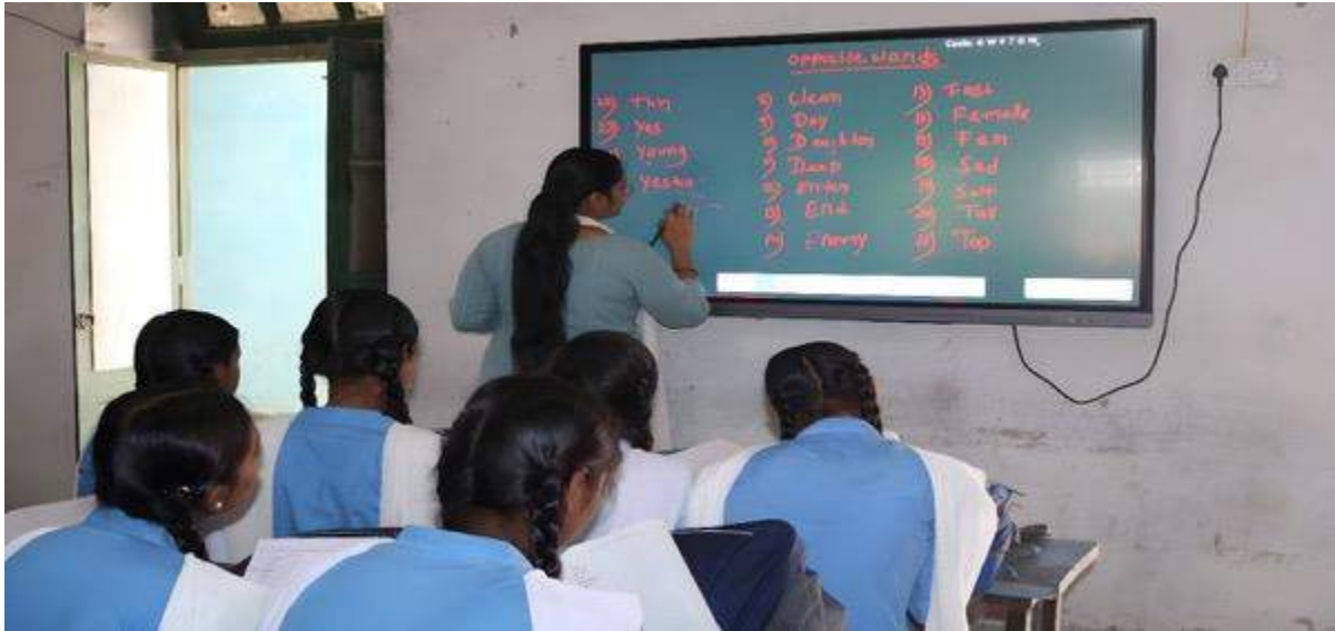
Fig: Supply & installation of Digital Board based Smart Classes at Govt. School, Bihar
