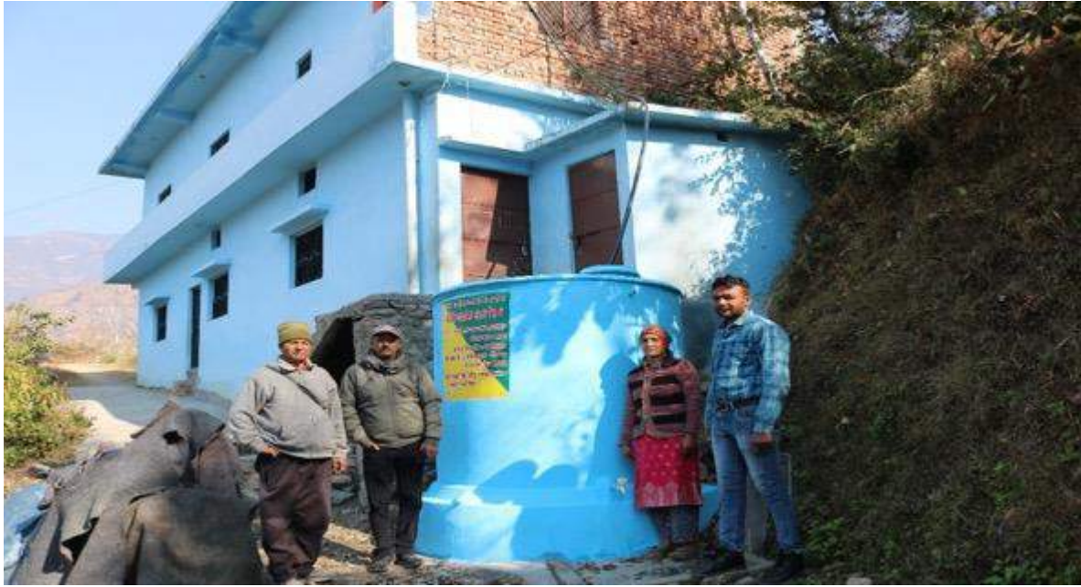
Fig: Construction of household roof rainwater harvesting tanks at Chamba, Tehri Garhwal
