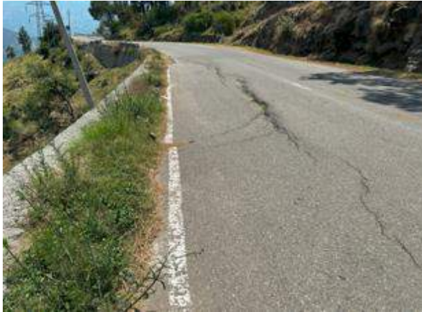
Fig. Initial subsidence observed on the Road
