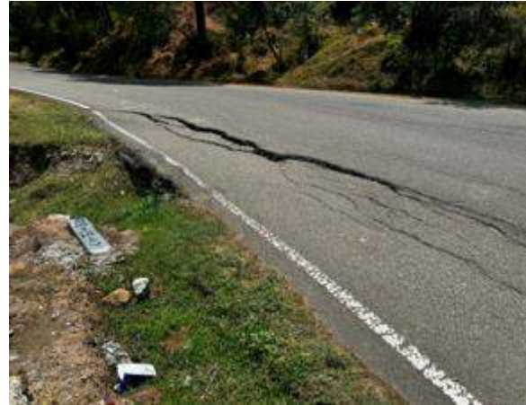
Fig. Prominent Cracks developed on the pavement
