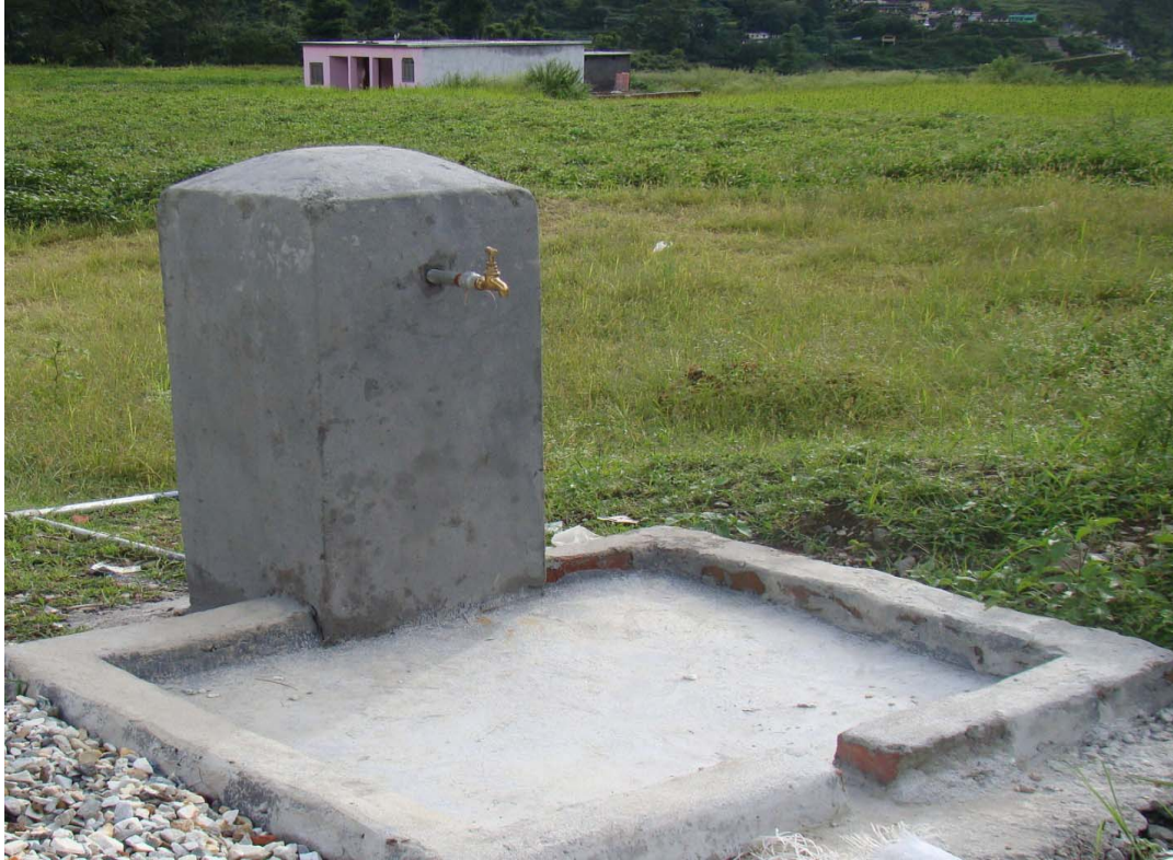
DRINKING WATER FACILITIES
