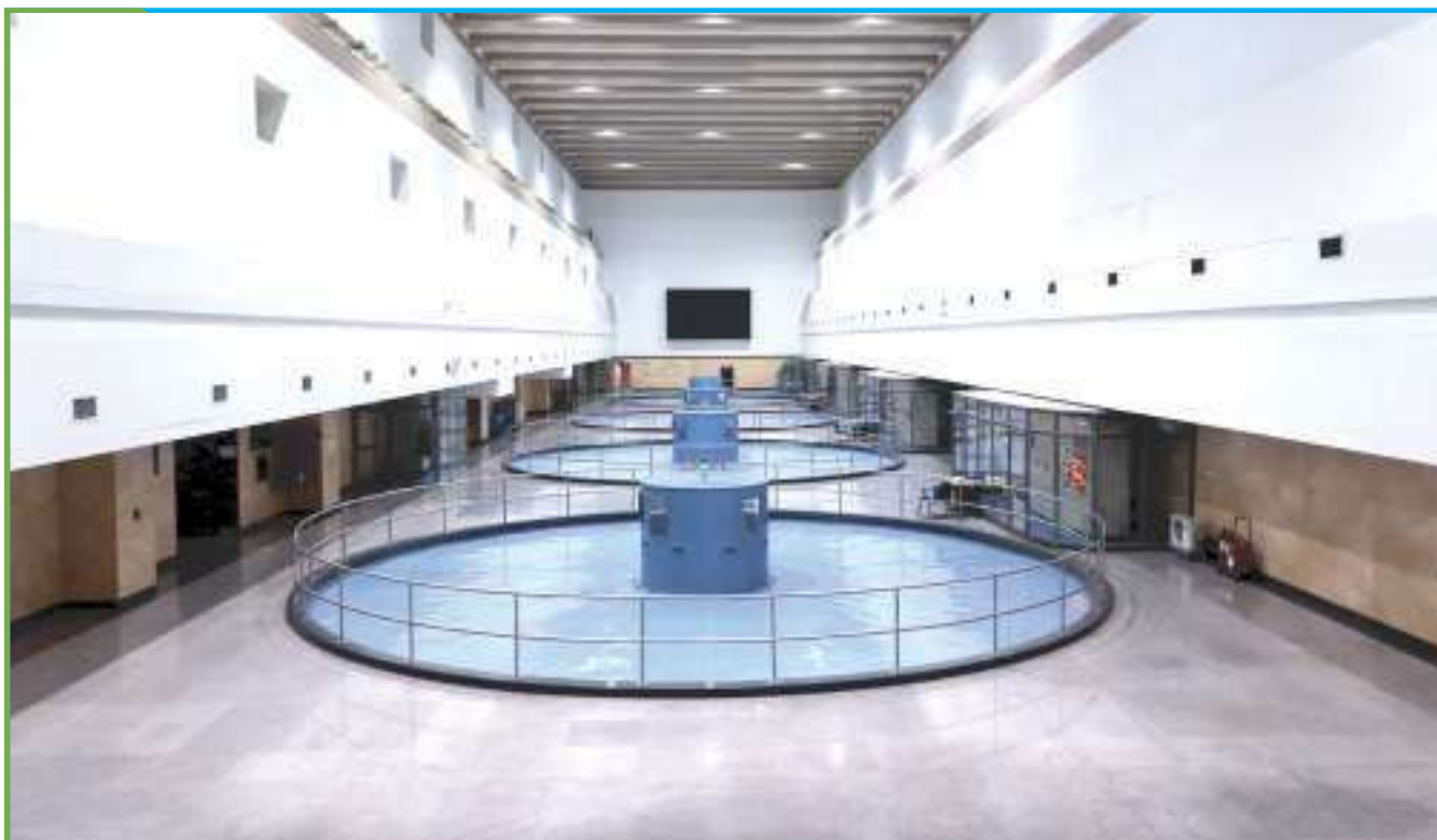
Power House of Koteswar HEP (4x100 MW) 400 MW
