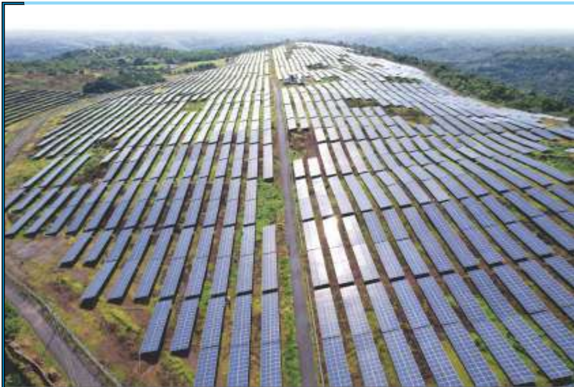
50 MW Solar Power project, Kasaragod, Kerala
