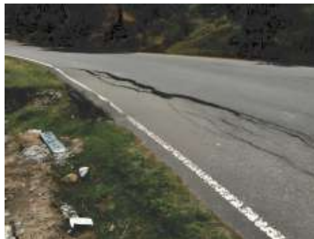
Fig.-8: Prominent Cracks developed on the pavement
