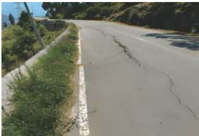
Fig.-7: Initial subsidence observed on the Road
